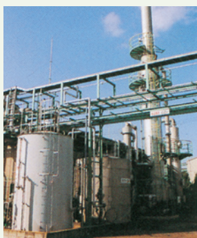
Waste liquid and exhaust gas incineration equipment at our Takaoka Plant
