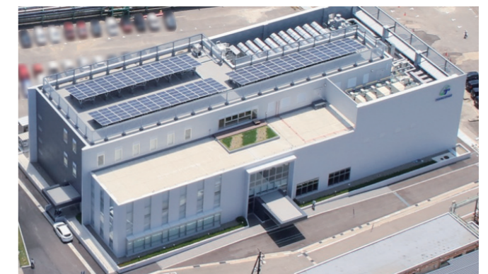
Rooftop solar power generation system (Takaoka Creation Lab)
