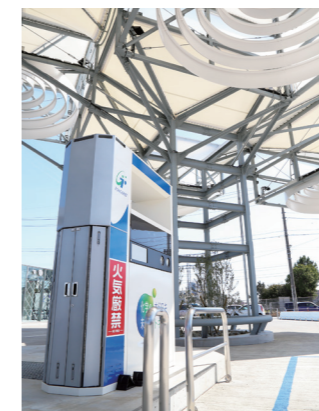
High pressure hydrogen dispenser
