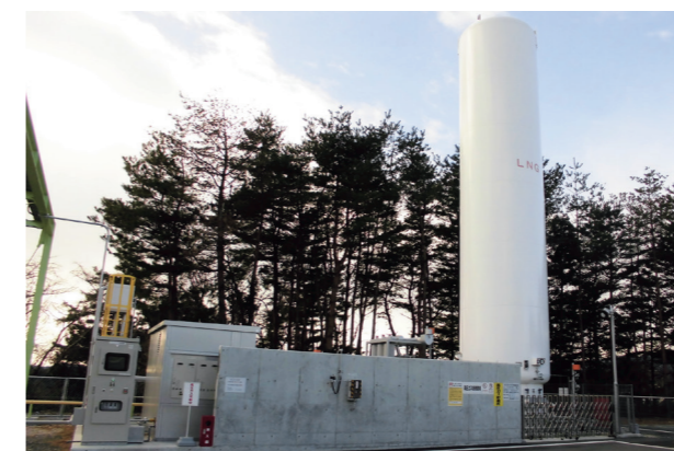
LNG Satellite Station for Hirono Plant Boilers
