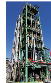
(New) hydrochloric acid facility at the Yokohama Plant
