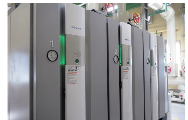
Takaoka Plant LNG Boiler Building
