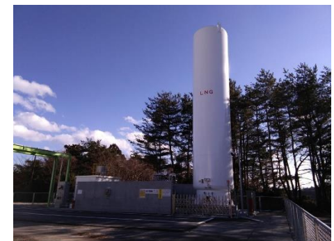
LNG facilities at Hirono Plant
